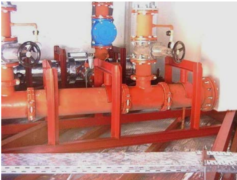
24" Dia Chilled Water Lines inside Pump Room
